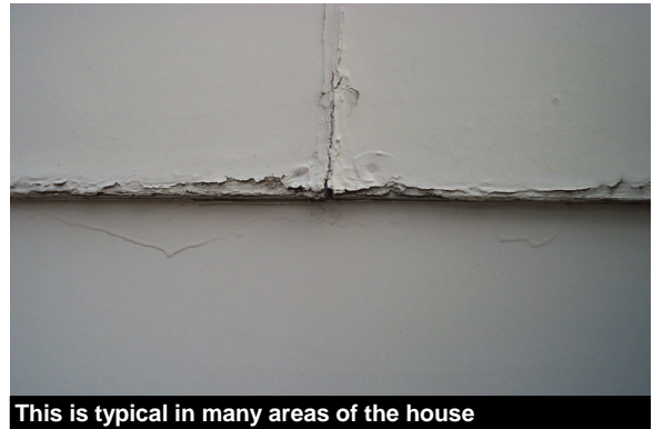
This is typical in many areas of the house
