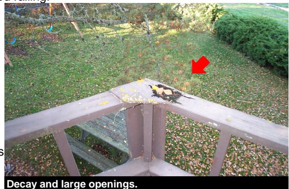
Decay and large openings.
