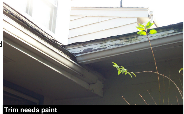
Trim needs paint
